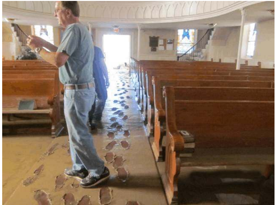
Flood damage at St. Mark's Lutheran Church in Middleburgh, N.Y., following Hurricane Irene.
