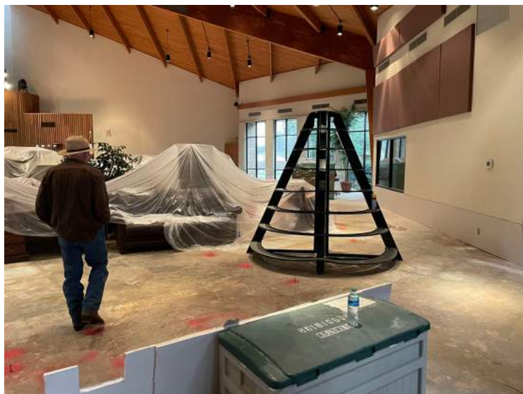
Flood damage at All Saints Lutheran Church in Arlington, Texas.
