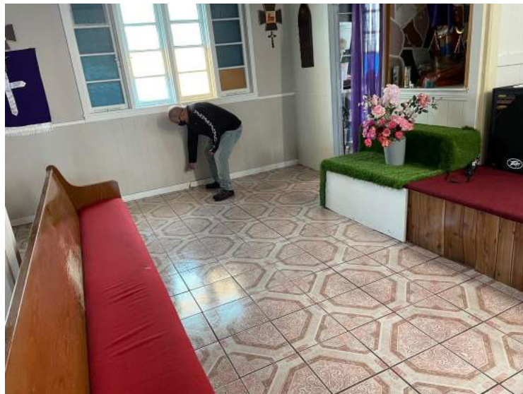
Pastor Juan Portillo showing the 12 inches of water that flooded San Miguel Lutheran Church in Fort Worth, Texas.
